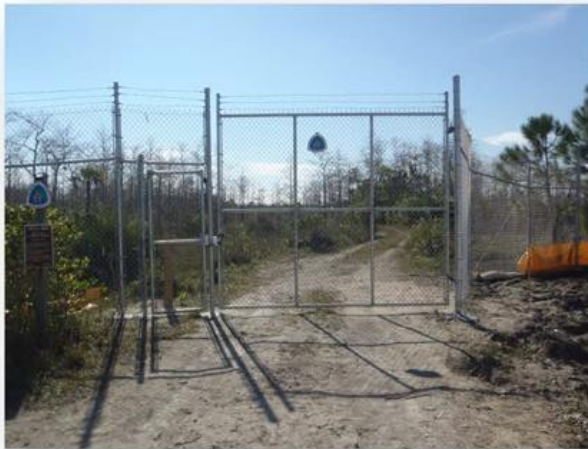
New gate from the south recreational parking construction into the Big Cypress National Preserve
